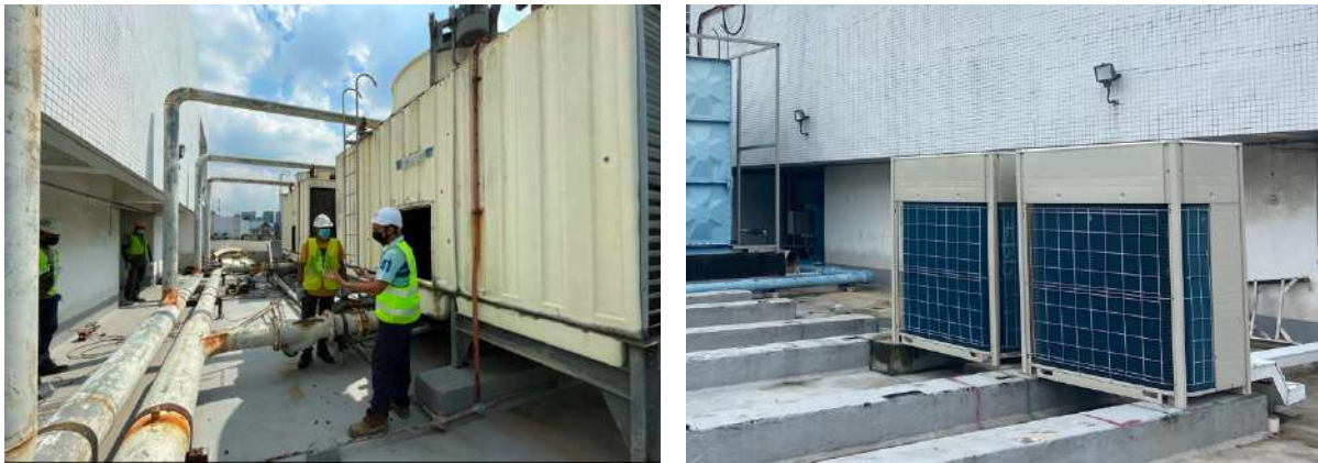
Figure 21 Dismantling of old cooling tower to replace with a more flexible and efficient VRF system
