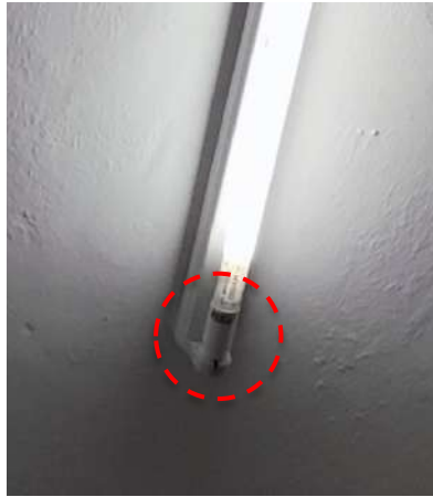
Figure 24 Retrofitted light fittings with built in motion sensor
