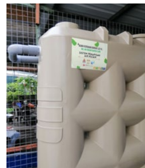
Rainwater harvesting system
